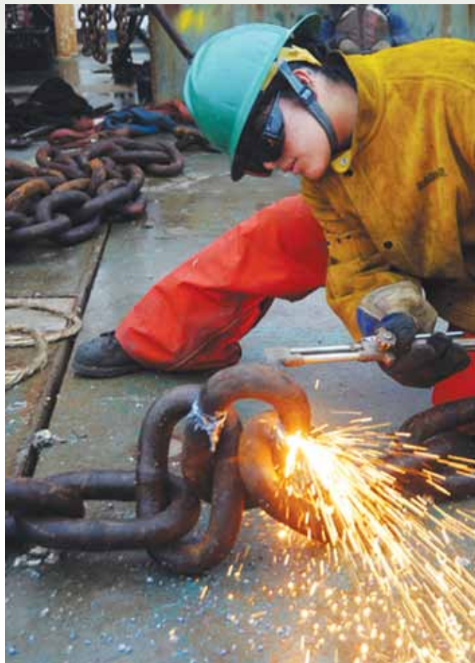
Seaman Alysia Orozco, a buoy deck rigger aboard the Aspen , cuts damaged chain off of a buoy using an oxyacetylene cutting torch.
